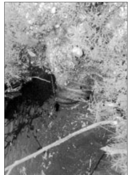
Rusting, eroding culvert on Algonquin logging road.
